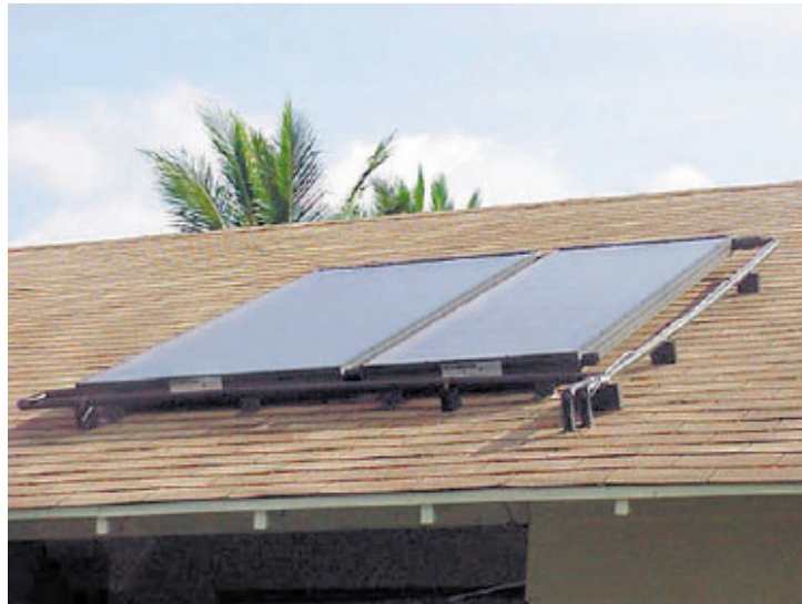
Figure A 2: Solar hot water collectors.
